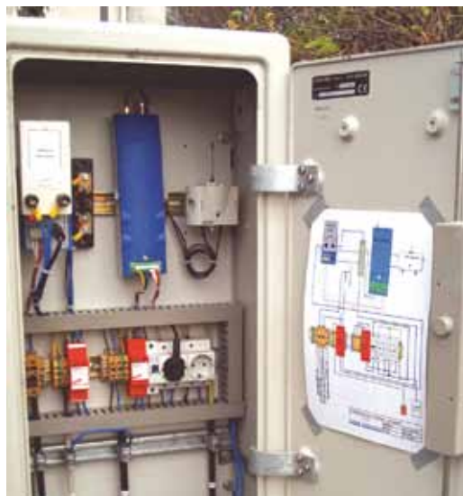
Remote controlled switching of rectifier system with mains power supply unit
