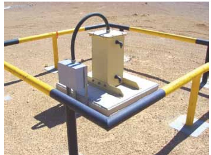
Steel support mounted AJB on concrete foundation at anode deep grounded structure (with crash barriers)
