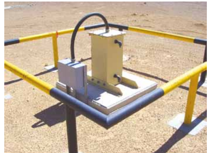
Steel support mounted AJB on concrete foundation at anode deep grounded structure (with crash barriers)
