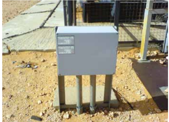
CJB with hot-dipped galvanised steel supports
