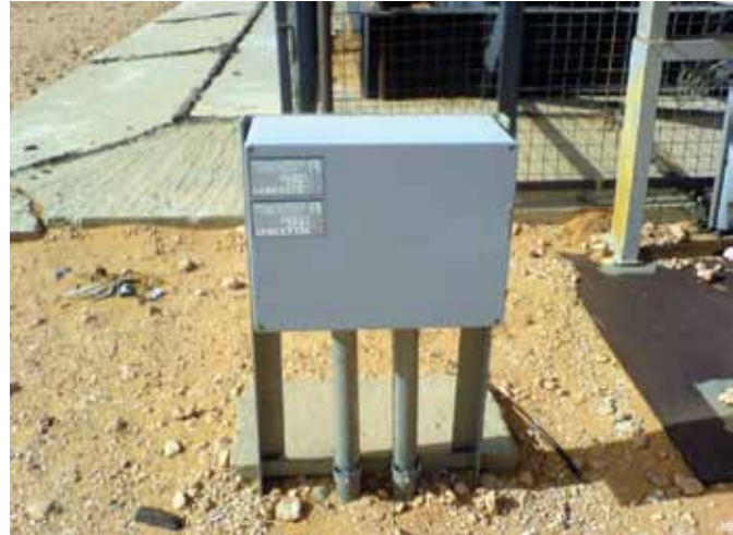
CJB with hot-dipped galvanised steel supports
